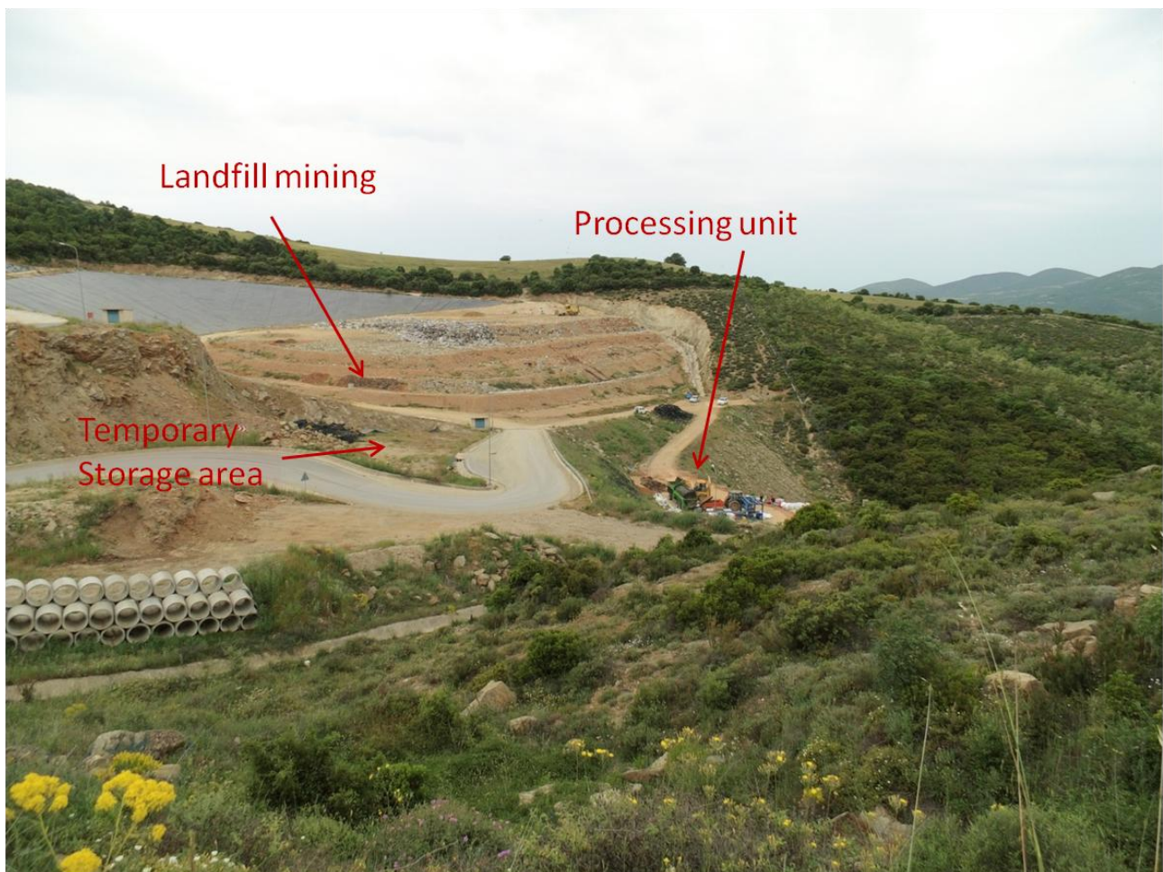
Figure 3: Sitting of the excavation, the processing unit and the temporary storage area
